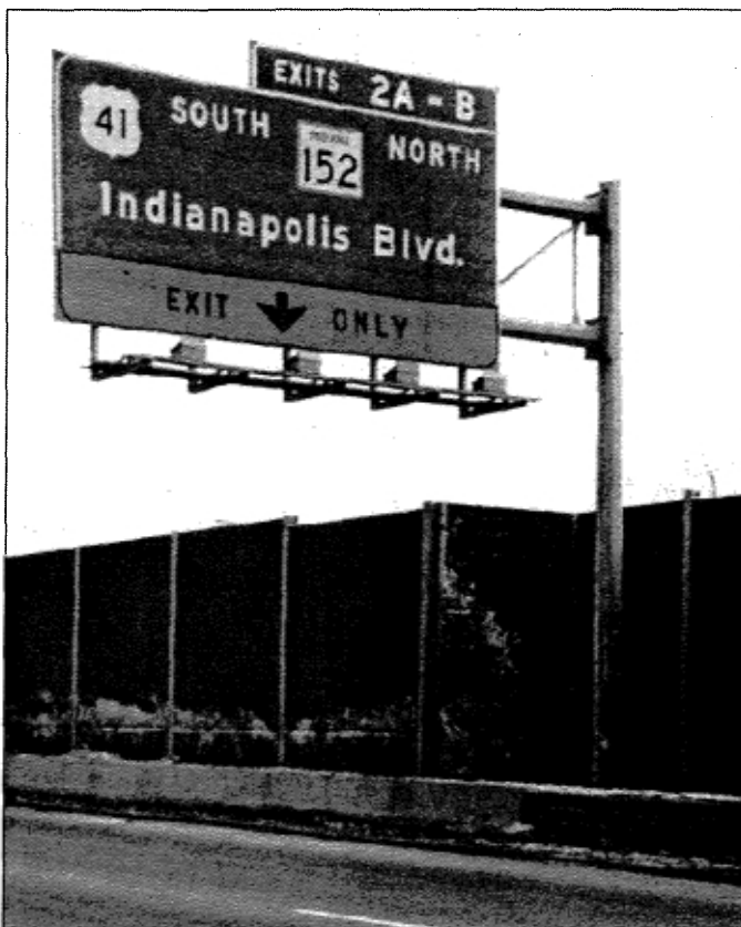
Traces of salt-laden snow deposited on sound barrier by truck traffic and snow plows are visible 16 feet above pavement on ground-mounted sound barrier 10 feet from the guide rail.
